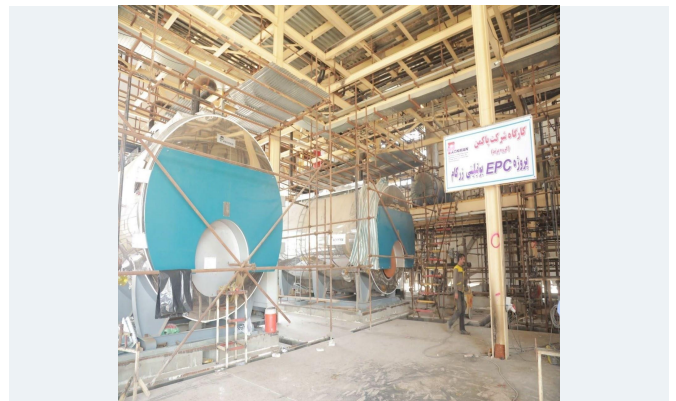
Boiler shell, platform and overhead pipework
