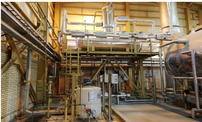
Installed equipment within a boiler hall
