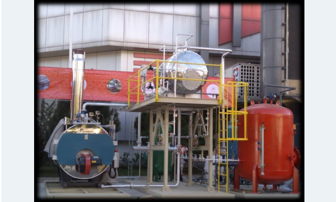
Boiler equipment and auxiliary vessels
