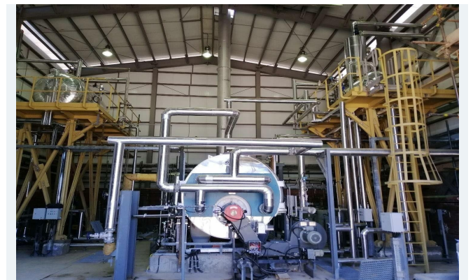
Boiler front and surrounding access structure
